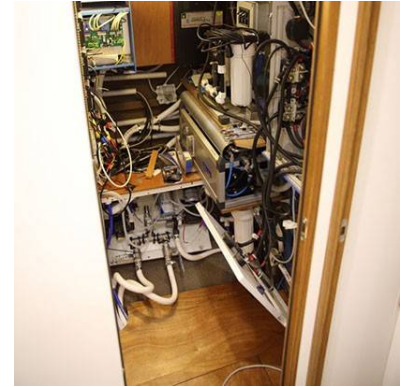
The technical room of the Gulliver 57.
